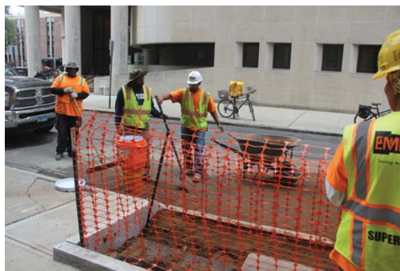
Workers from Emerge Connecticut Inc. construct a bioswale near the intersection of Wall and Church streets in New Haven in October.
